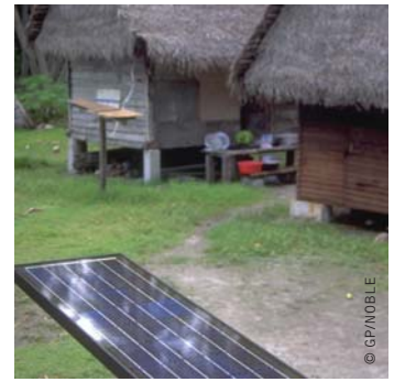
image PHOTOVOLTAIC (SOLAR) PANEL ON TOBI ISLAND, BELAU ISLANDS, PACIFIC. THESE PANELS PRODUCE ALL THE ELECTRICITY USED ON TOBI ISLAND.
